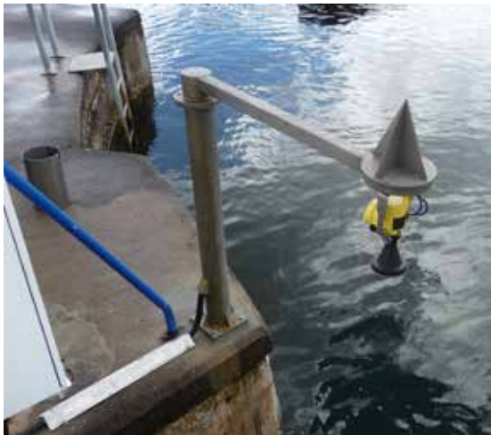
Figure 7. Typical Radar Station (Jervis Bay)
